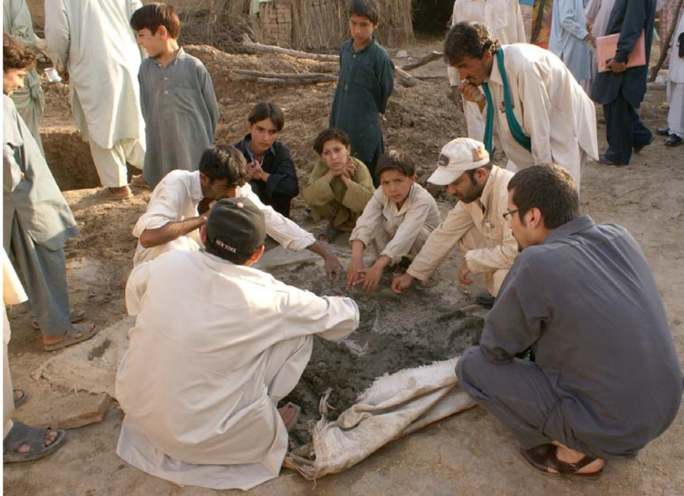
Boys take interest in the construction of latrines as CWS-P/A and partner staff inspect the quality of the cement mixture, photographed by CWS-P/A staff
