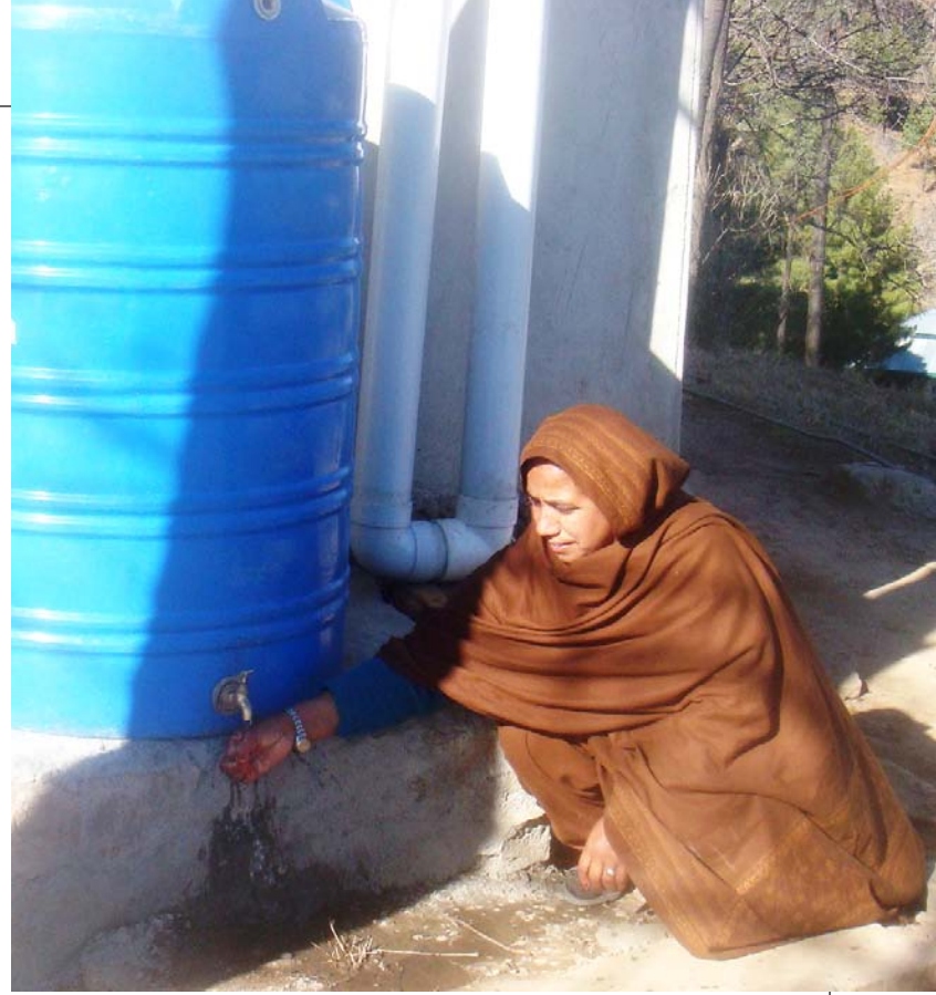
Ruqia Begum demonstrates use of the rainwater harvesting system, photographed by CWS-P/A staff
